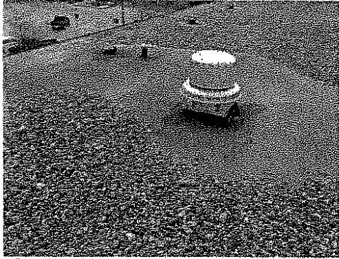
Small RTU fan, plumbing stack, and pitch box.
