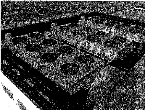
Roof measures 27'x40' FA EPDM with a through wall scupper in the southwest corner
